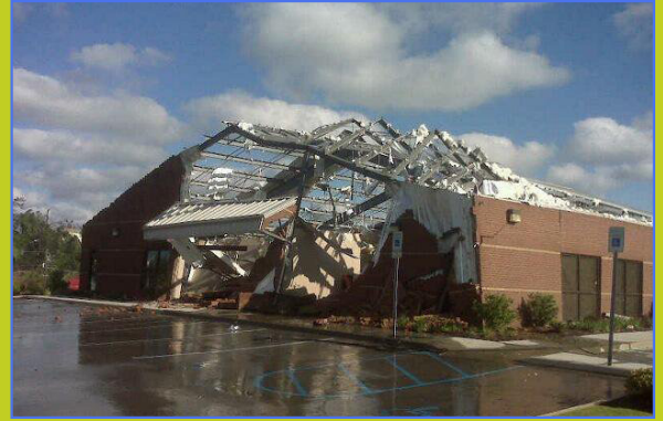
Alabama 811's call center after the tornado hit it on April 27, 2011
